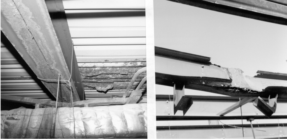
Figure (4) Corrosion of steel joist before (left) and after dismantling the floor (right).
